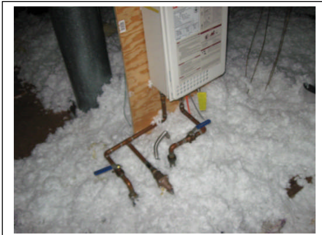
Picture 7 Missing water heater safety pan
