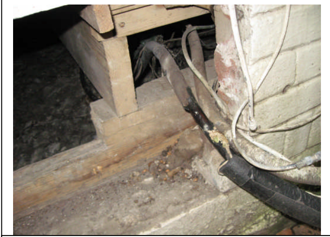
Picture 4 Missing Freon line insulation
