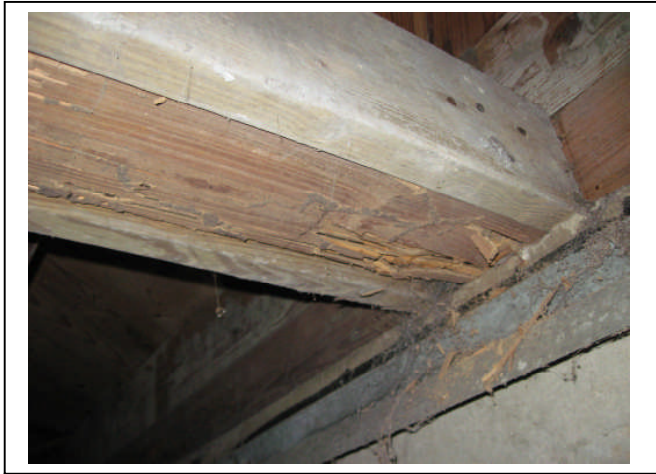
Picture 5 Front sub-floor damaged beam
