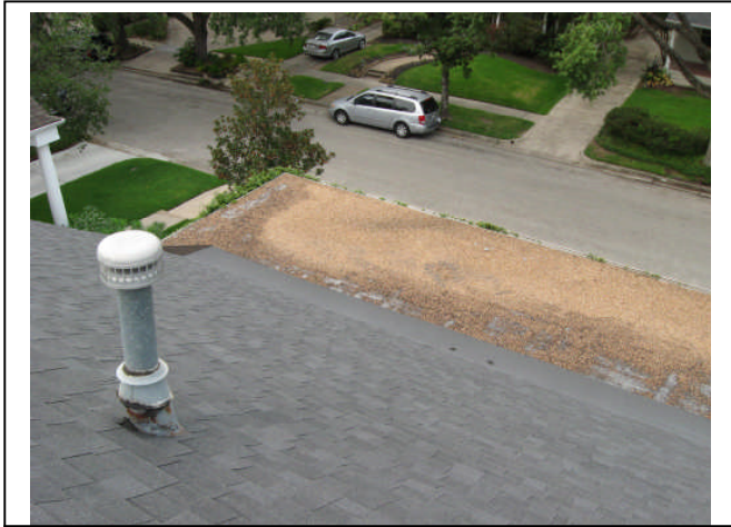
Picture 8 Front roof exposed membrane
