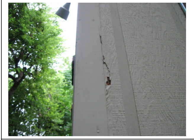
Picture 3 Living area chimney wood rot
